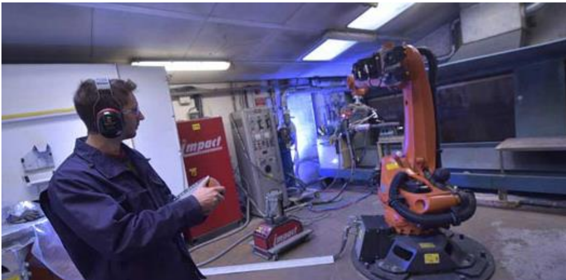
Figure II. 6 : Installation cold spray "haute pression" installée chez Mallard.
