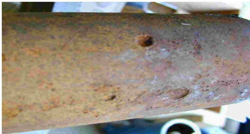
Figure III. 6 Corrosion externe (Pitting d'un pipe).
