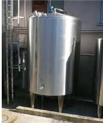
Figure 2 : Tank de stockage
