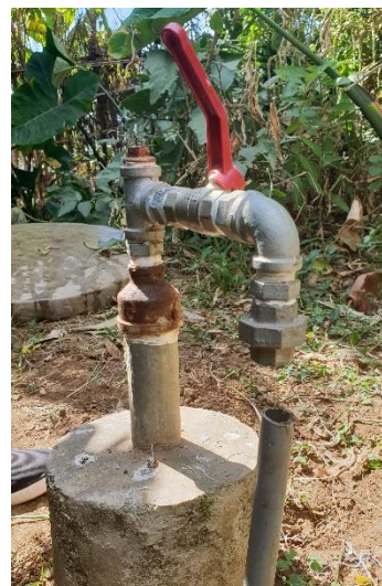
Fig.2: dome outlet valve. Only a small amount of biogas was exhausted when it was opened.
