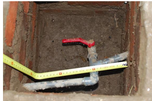
Figure 4: purge valve that should be open every day at least few seconds.
