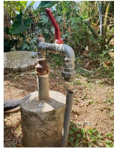
Figure 3: gas tap should be carefully controlled, due to the several joints on it.
