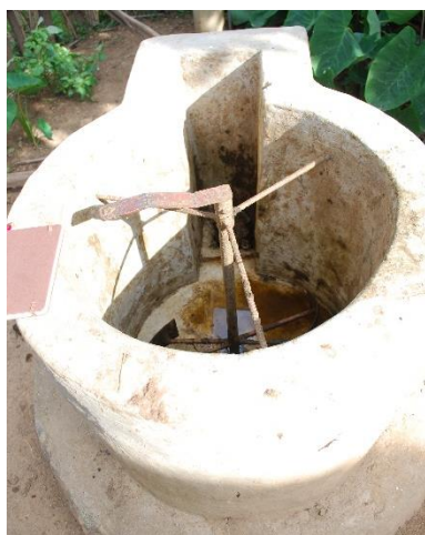
Figure 1: feed chamber, where feed is added every 2 days. Stirring is used to mix the feed before it enters the digester.
