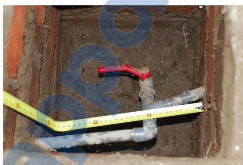
Figure 1: biogas tap, allowing the evacuation of condensated water in pipes.
