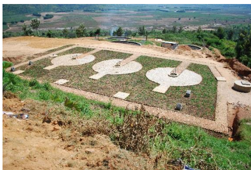
Figure 3 : 3x100m 3 digesters, built during phase 3 of construction, due to the increasing number of inmates in the prison.
