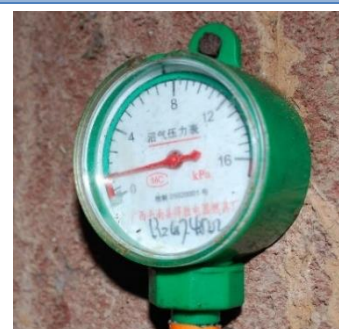
Figure 3: digester's pressure manometer.
