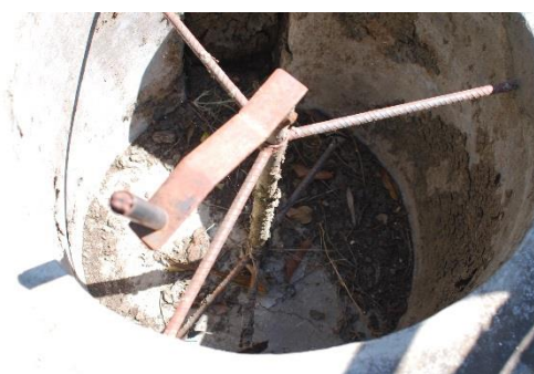
Figure 2: stirring equipment where rust should be removed before rehabilitation.
