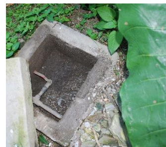
Figure 4: condensate tab to remove water from gas pipes.
