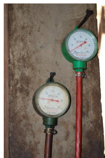
Figure 4 : manometer, used to measure biogas pressure. According to the person in charge, the outlet pressure can reach 15 to 16 kPa
