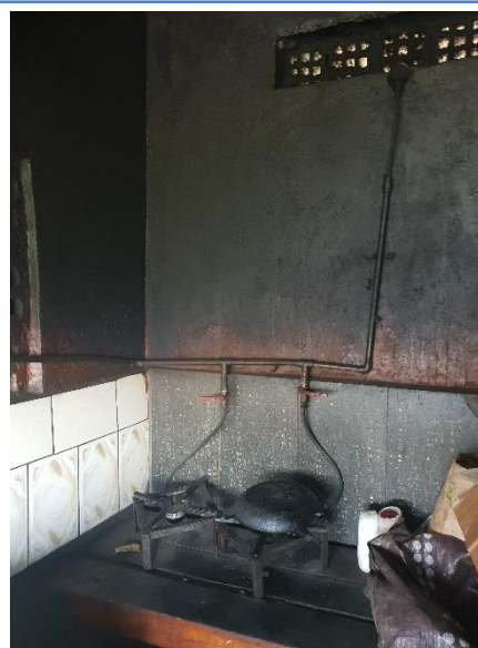
Figure 1: biogas pipes, where two stoves are still connected but not currently in use. A manometer is visible up right.
