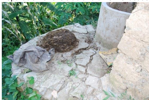
Figure 3 : slab that can be repaired near the feed chamber.
