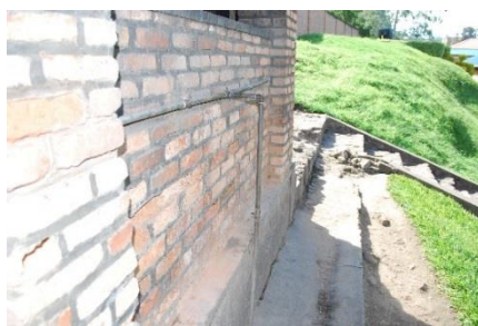
Figure 3: pipes used for the biogas in front of the kitchen.
