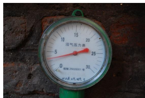
Figure 6: manometer used for the 4x100m 3 digesters. According to the person in charge, pressure can reach about 12 kPa.
