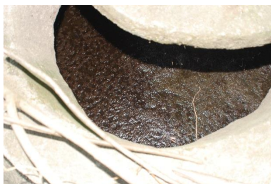
Figure 3: slurry in evacuation chamber (and probably digestion chamber) that should be removed before rehabilitation.
