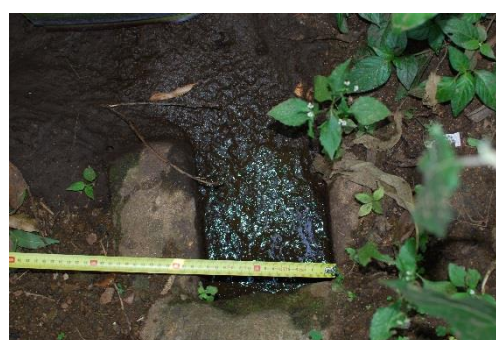
Figure 2: slurry exit from evacuation chamber.
