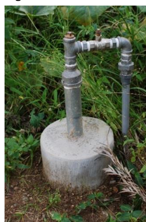
Figure 2: biogas exit from digestion chamber.
