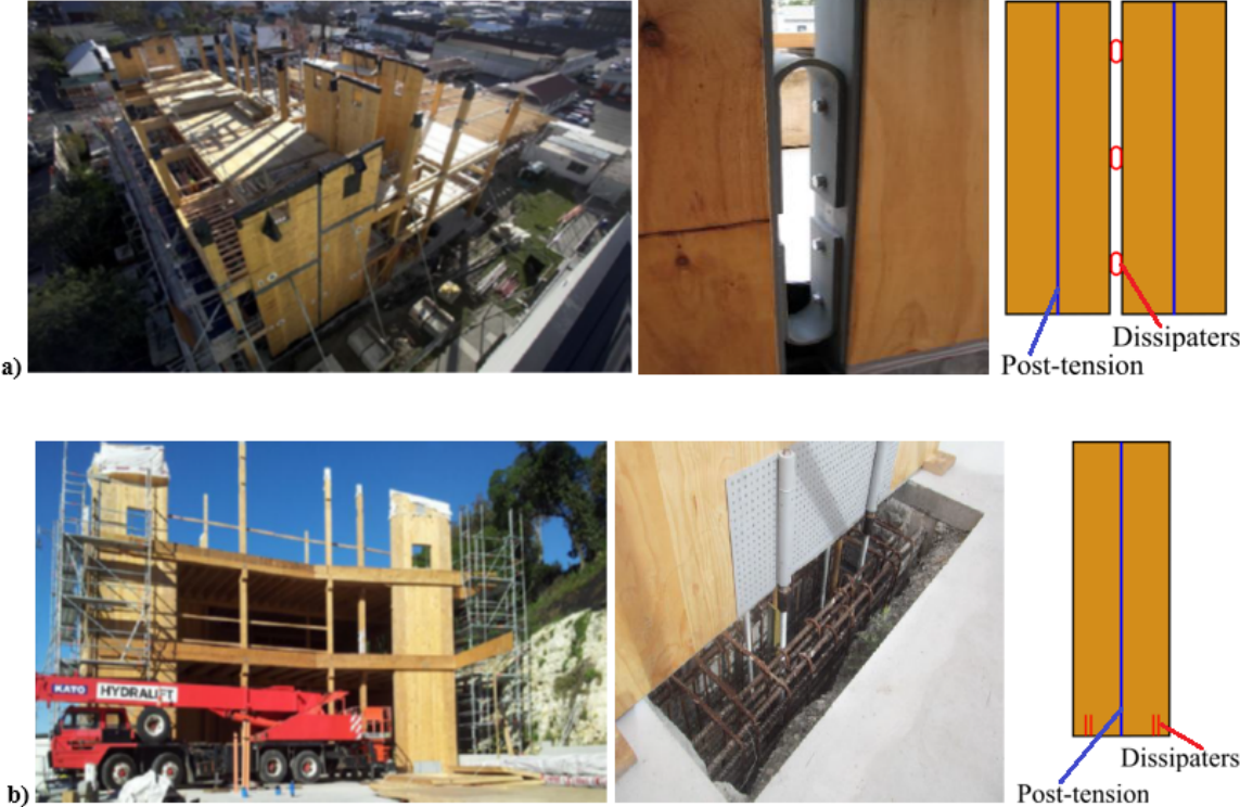
FIGURE 2.2 – Buildings and systems examples. (a) Nelson and Marlborough Institute of Technology. Coupled walls (adapted from Sarti, 2015) (b) Kaikoura District Council Building. Single walls (adapted from Sarti, 2015)
