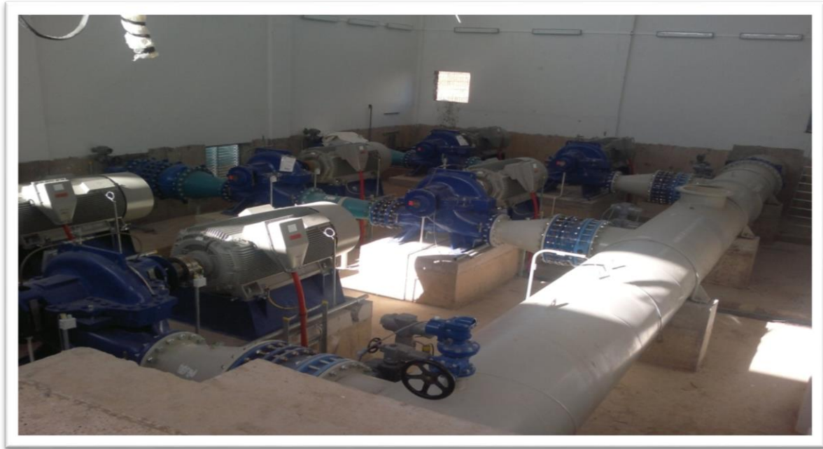
Photo II.6 station de pompage HSP2 [31]
