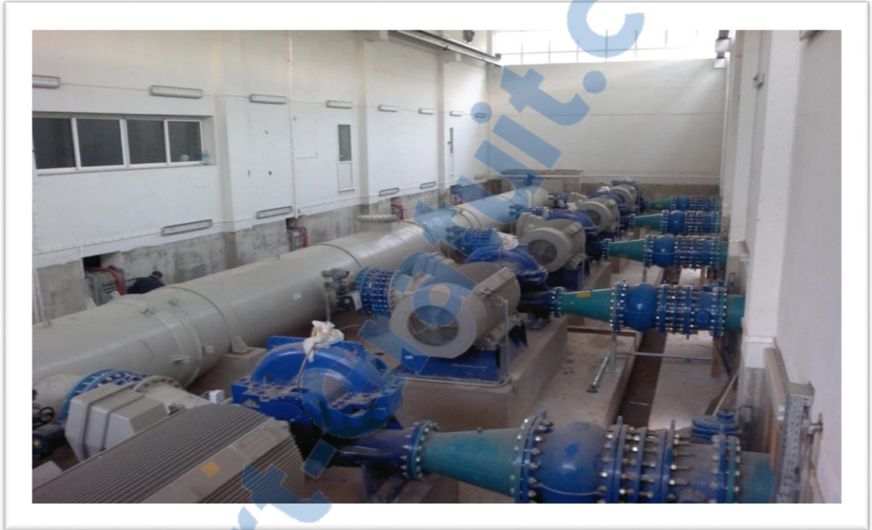
Photo II.4 Installation des pompes HSP1 [27]
