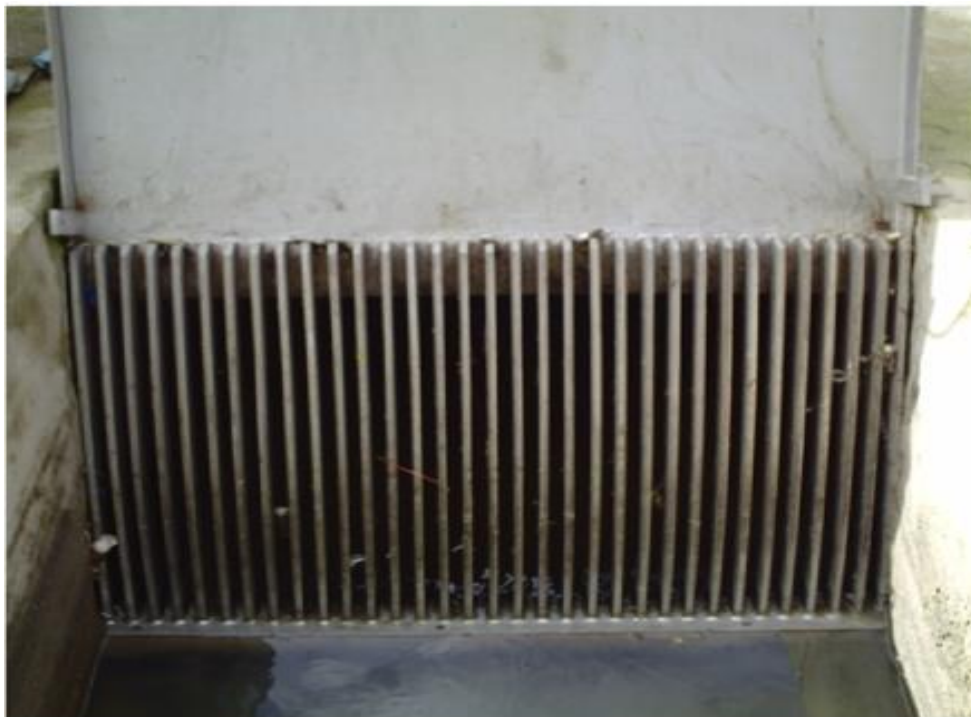
Figure III.6 : Photo de la grille fine manuelle de by-pass.
