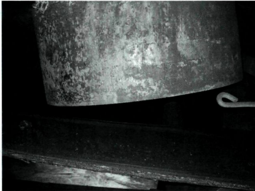
Figure 4.23 The iron-separator (after clean-up)
