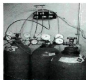
Figure 3.11 Carrier gas cylinders
